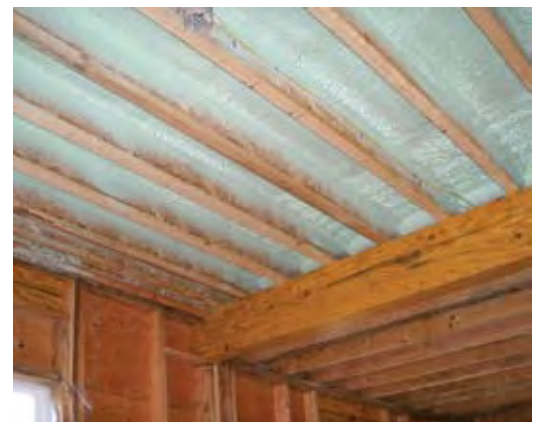
R-6 closed cell spray foam flash seal
